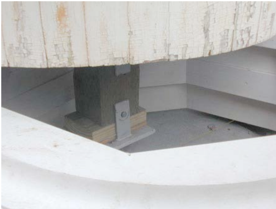
Figure 38: The base is centered. Note the cleats further securing the interior post. Where possible connectors were used to graft new pieces to existing posts.
