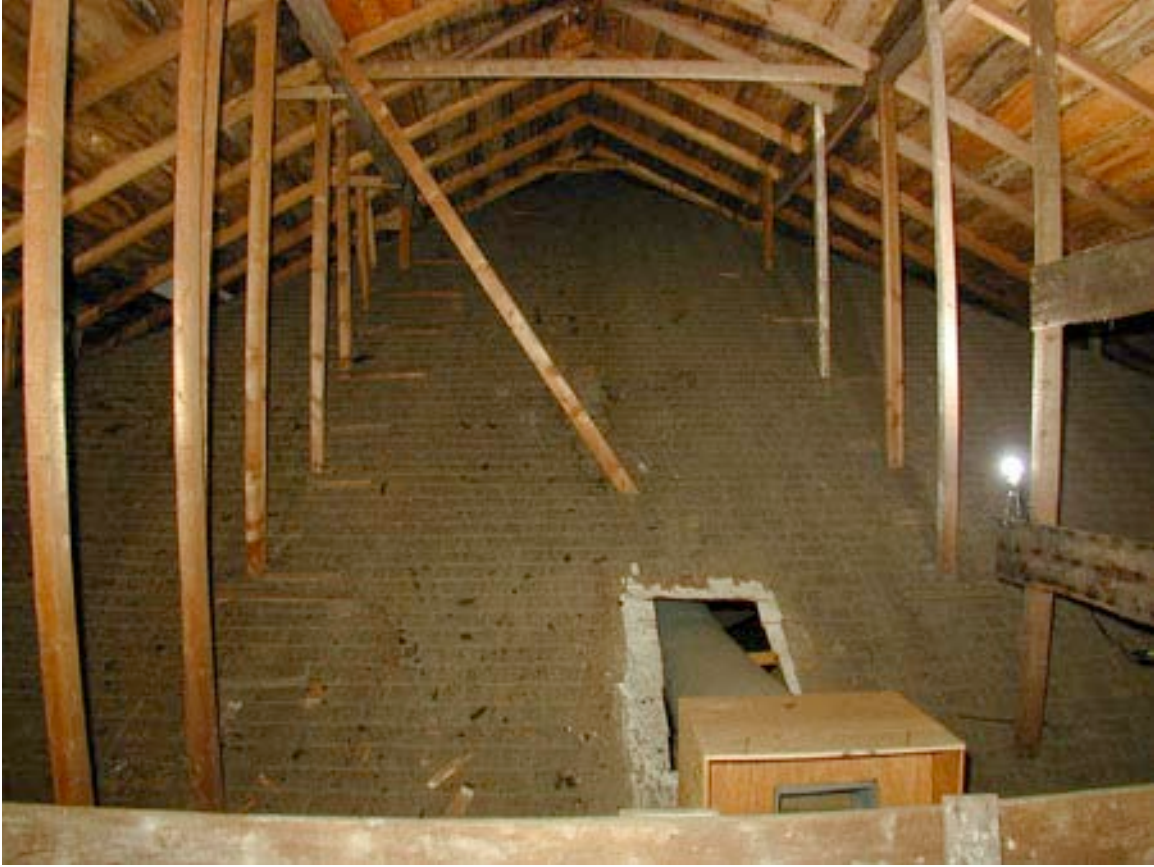
Figure 2: undersized members are inadequate to support gable. Columns are taking the weight.
