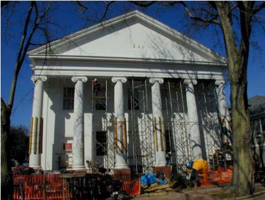
Figure 44: Progress continued on the façade until all columns could resume their loads.
