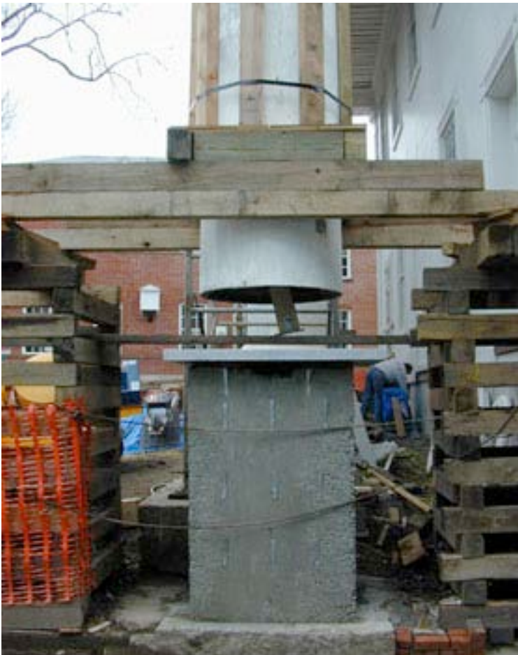
Figure 32: While the column is still suspended, 6X6 wooden support is positioned within the column for further stability and to prevent the load from sitting on the historic column itself. The granite slab is temporarily placed on top of the footing.
