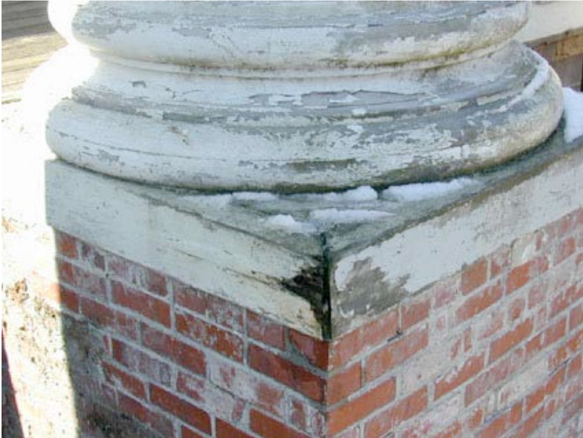
Figure 8: Water infiltration through columns has rotted wood bases
