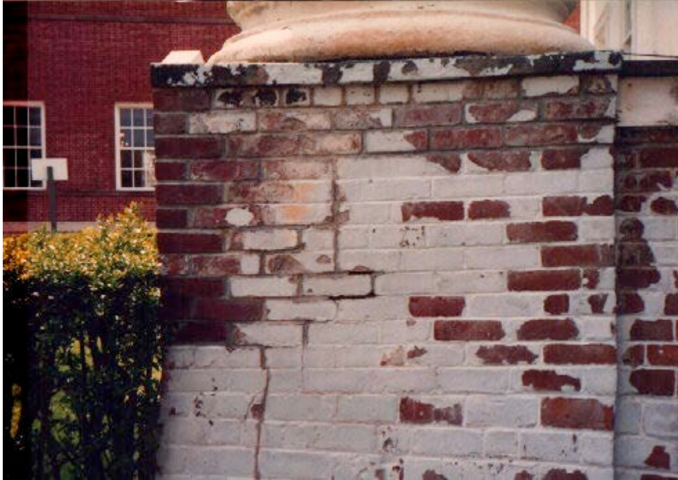
Figure 10: Partly crushed and missing bricks lead to a closer examination of causes.
