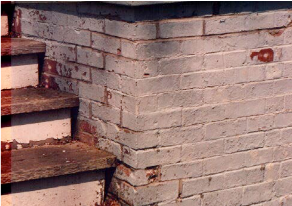
Figure 11: Detail of conditions found
