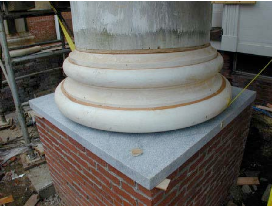
Figure 39: Here is a mock up of the final pedestal and base system. Note that the base is made in three pieces and that it is suspended until the final positioning of the granite cap.
