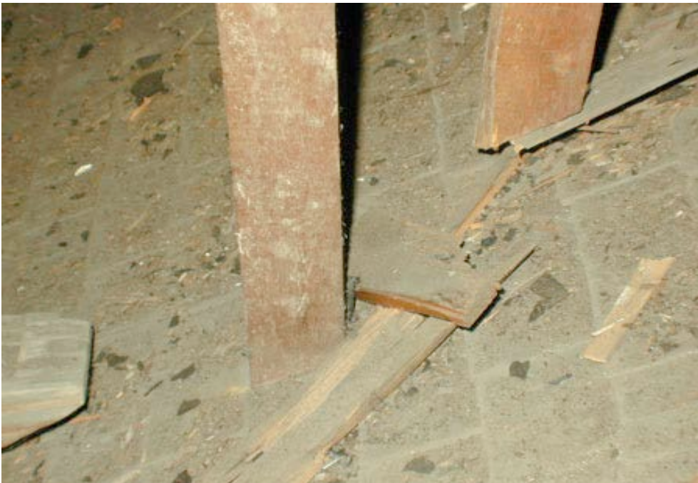
Figure 3: Detail of poor construction methods
