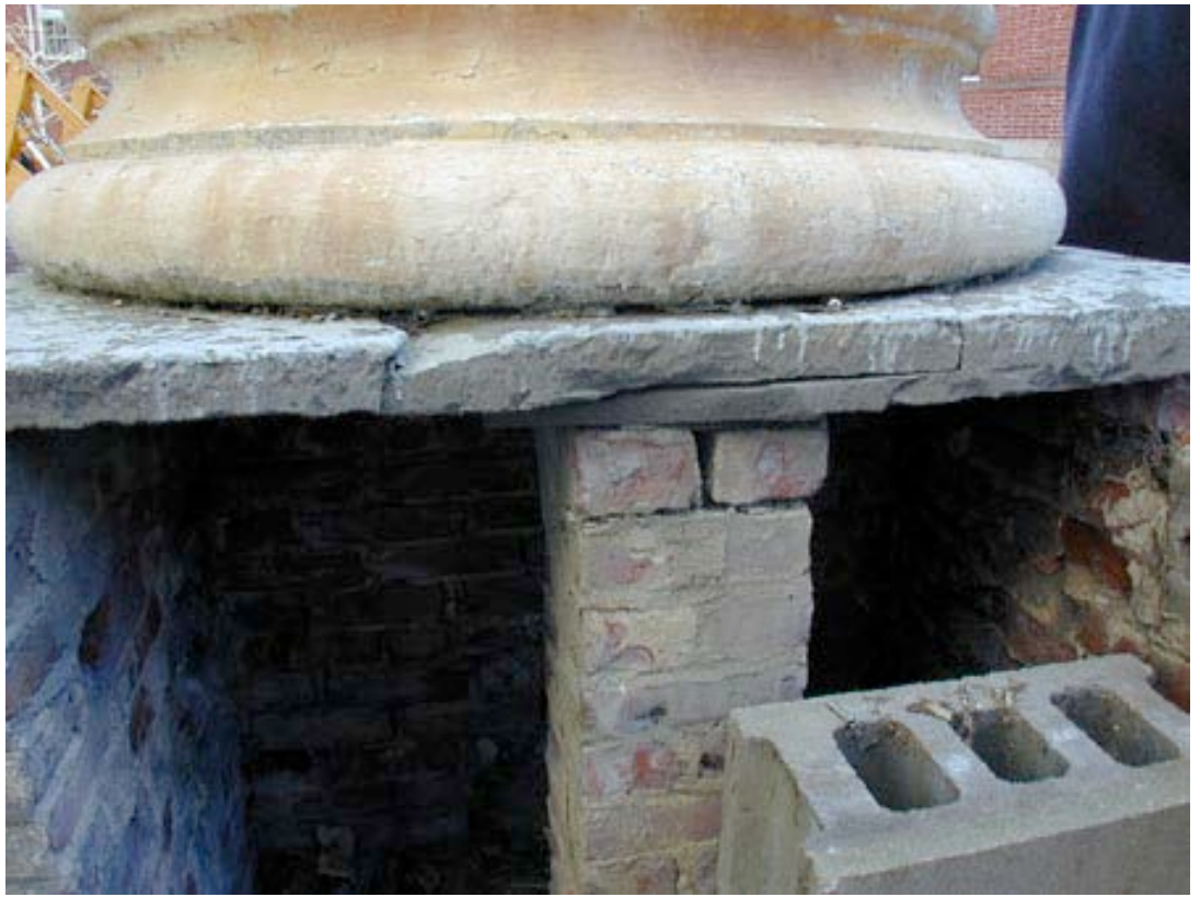
Figure 19: Stone base is cracked and brick support is failed
