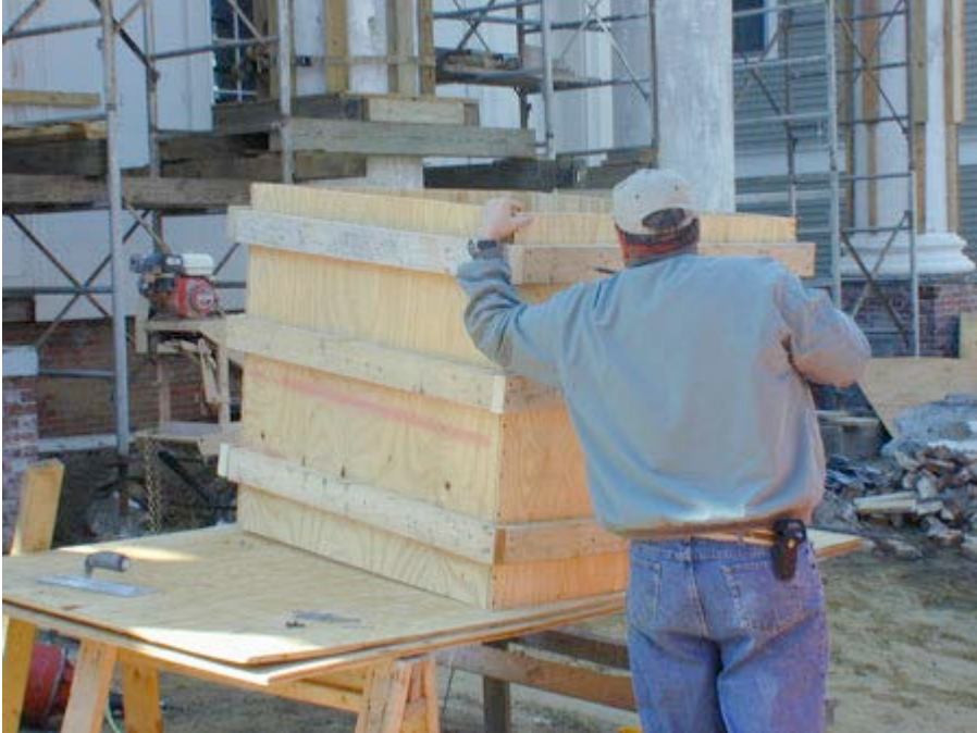
Figure 29: A form was created for each of the pedestals. This was secured with steel straps
