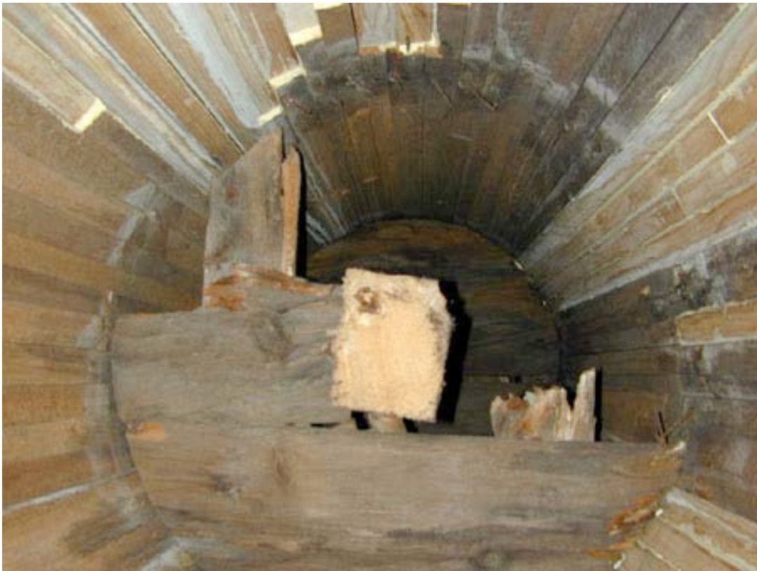
Figure 20: Looking up inside column, no more support
