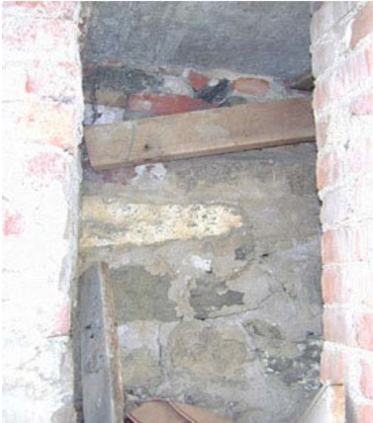
Figure 15: Inspection reveals columns supported by rubble. It turned out also that only 3 columns has central post supports remaining.
