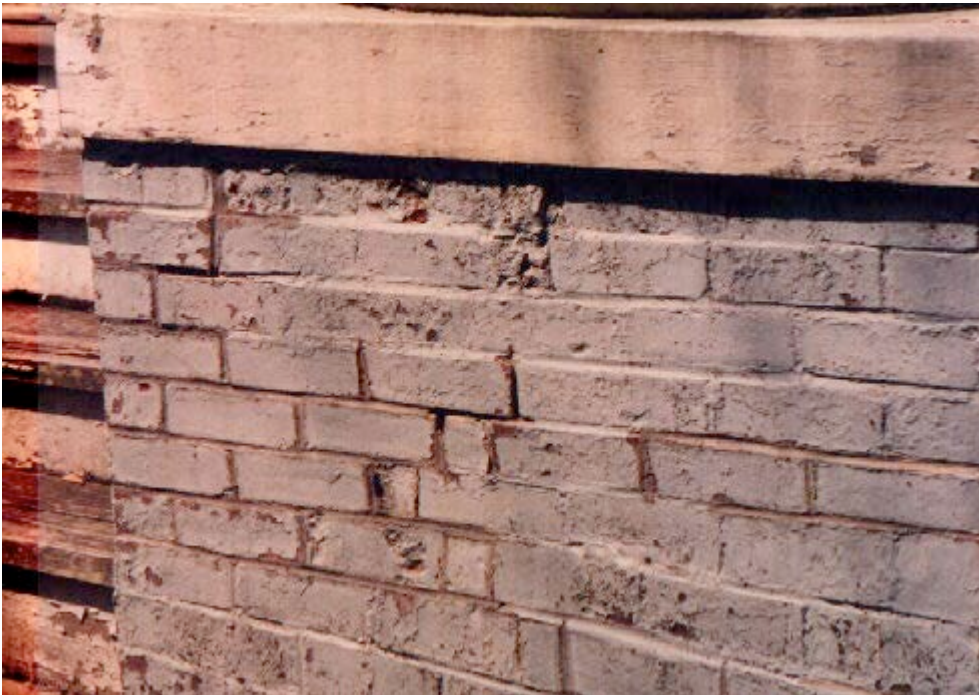
Figure 7: Missing mortar and cracking are the result of loading
