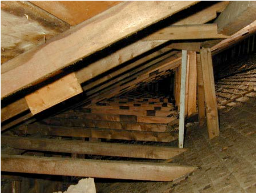
Figure 5: Here undersized outriggers struggle under their loads
