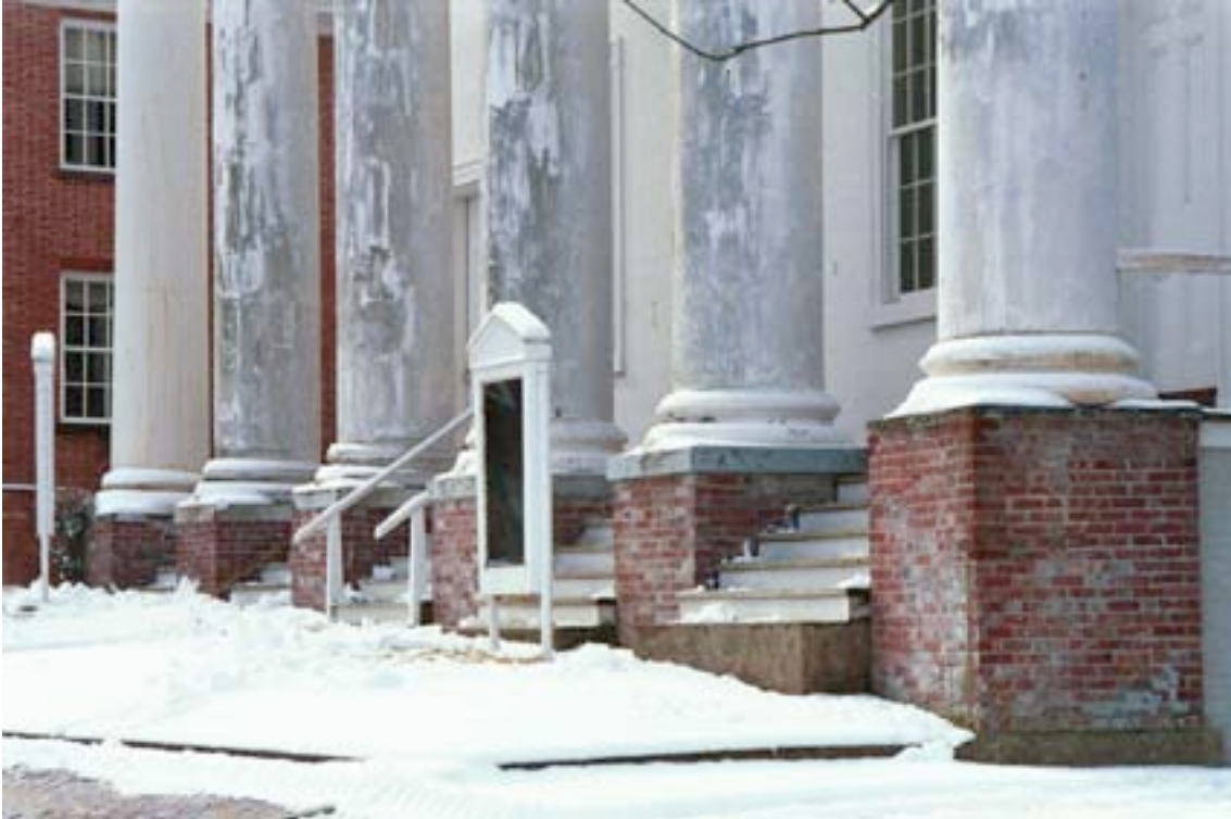
Figure 6: General conditions of bases prior to Phase II
