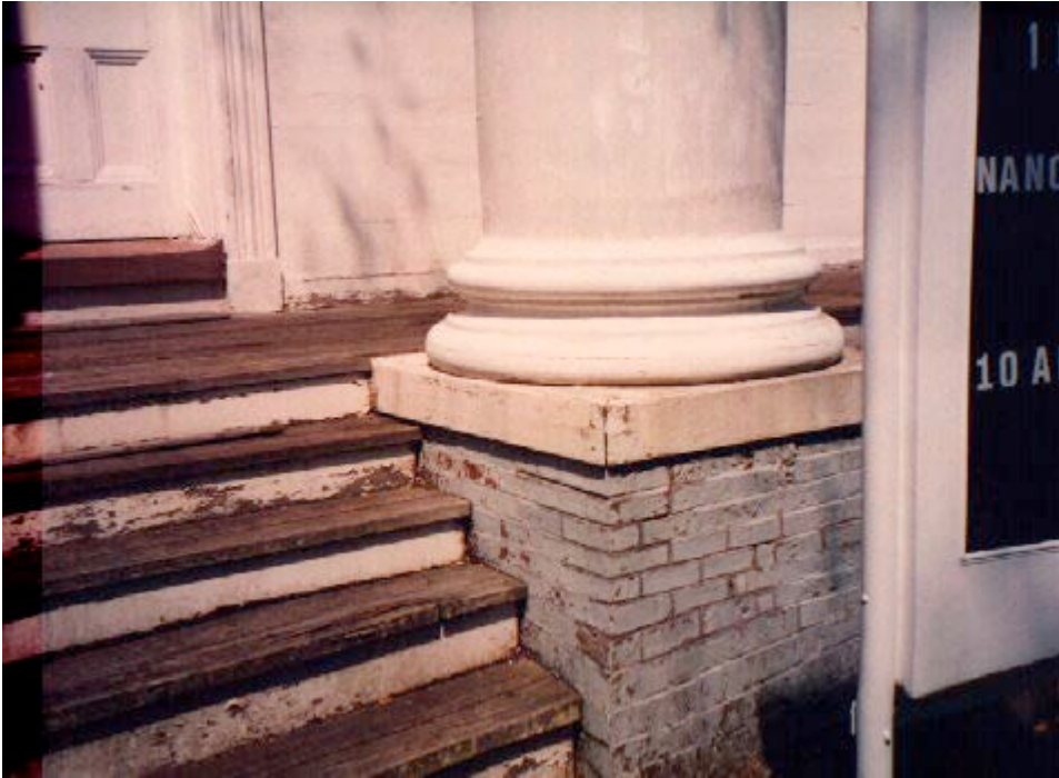
Figure 9: Detail of masonry failures, fungal and mold growth and bad mortar match
